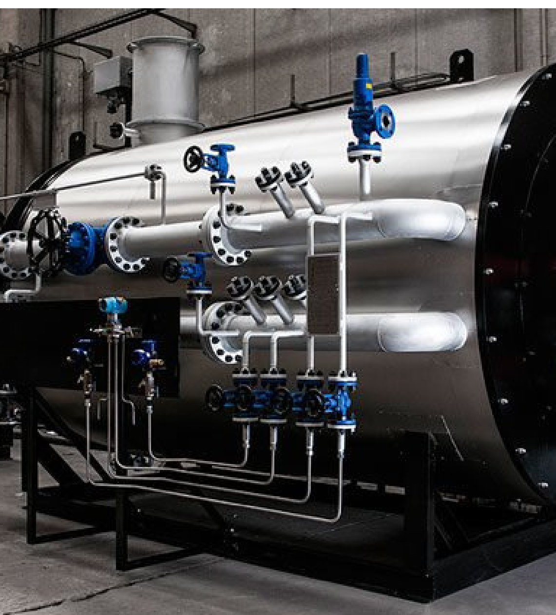
Thermic fluid system
